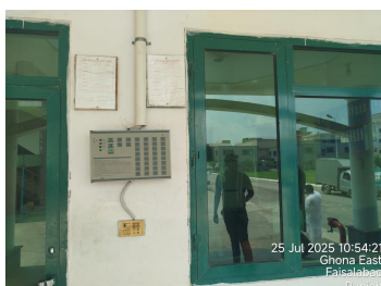
6. Centralised fire alarm system.jpg
